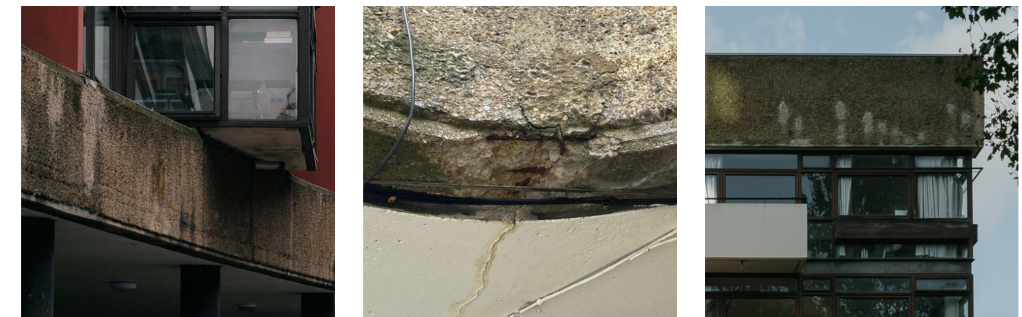
Bushhammered concrete showing signs of staining, spalling and sub-standard historic repairs
