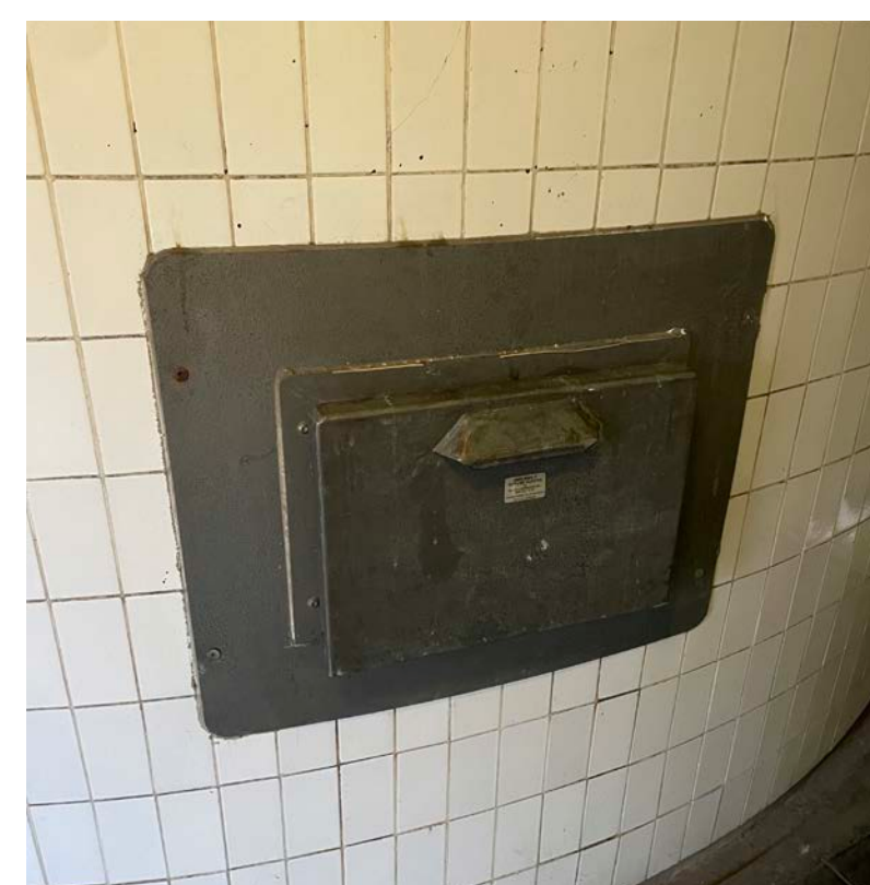
Existing refuse chute hopper
