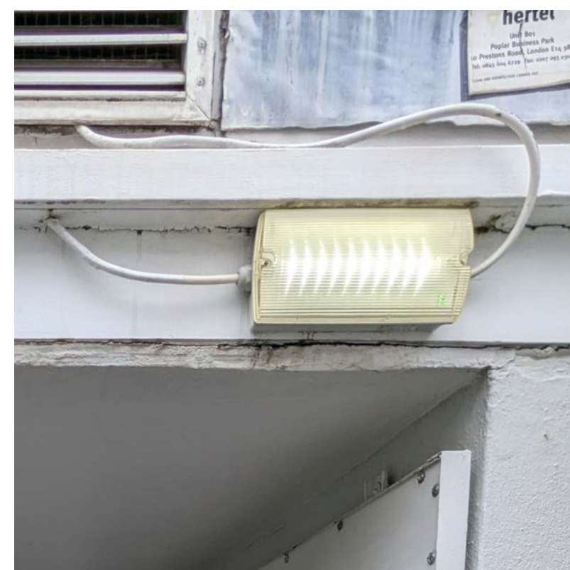
Light fitting in external corridor
