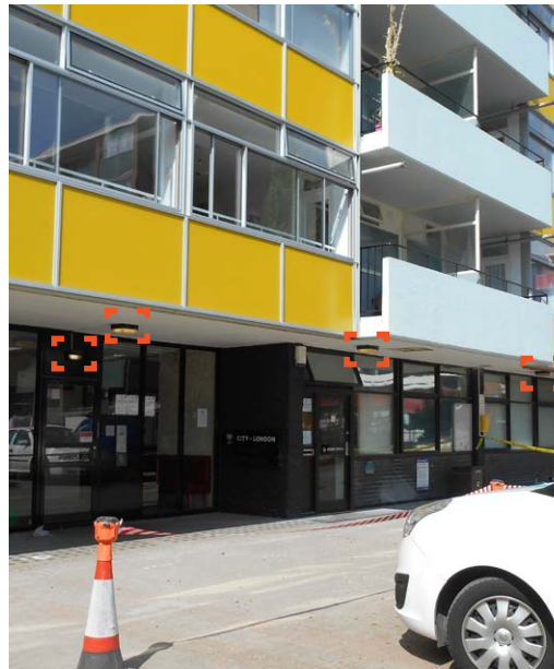
Great Arthur House- Eastern facade. Fittings cat. 2 and cat. 9. Installed in 2018 (Agreed by CoL Planning Dep.)
