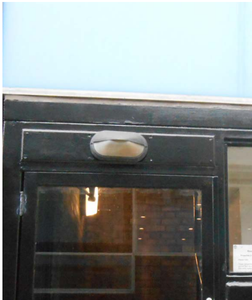
External fittings above the entrance to Bowater House. Fitting cat. 10.
