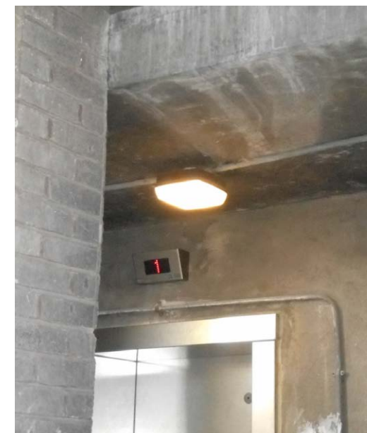
Garage lighting. Fittings cat. 21.
