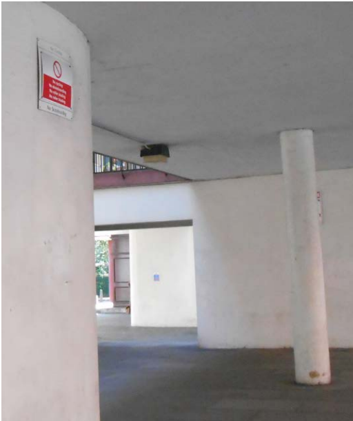
View looking in to east of Crescent House. Fitting cat. 2.
