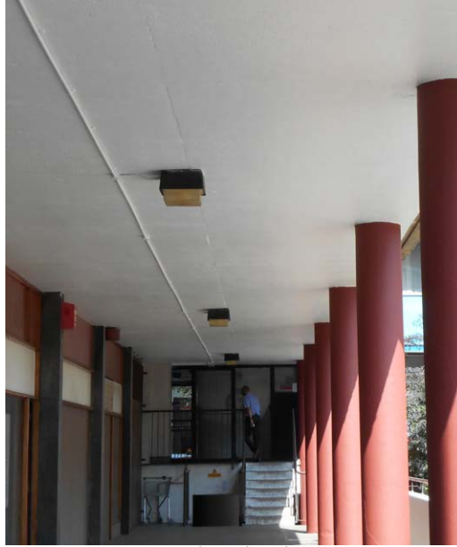
Crescent House, Podium level. Fittings cat. 11.
