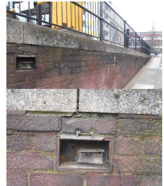
External fittings on a retain wall next to the Bowater House. Cat. 25.
