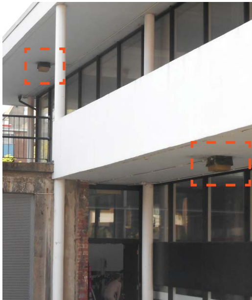
Leisure Centre, walkway lighting. Fittings cat. 2.
