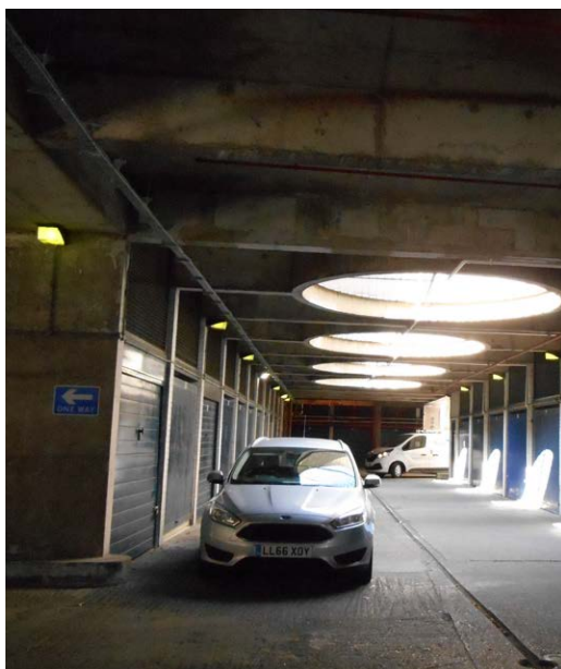
Garage lighting. 12 Fittings cat. 5.
