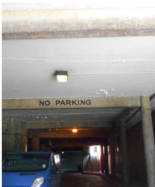
Garage lighting. Fittings cat. 2.
