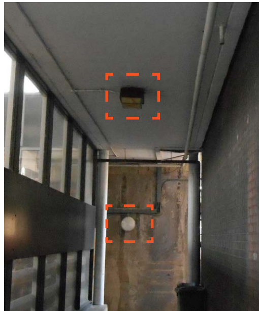
View looking south. Fittings cat. 2 and cat 19.
