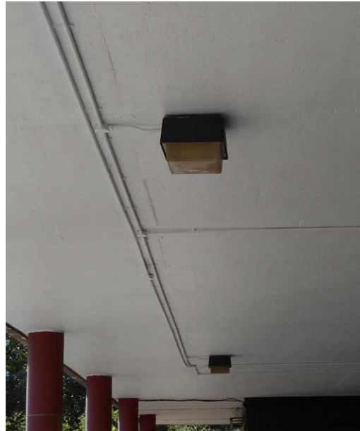
Lights in the ceiling, view looking onto Fann Street. Fitting cat. 2.
