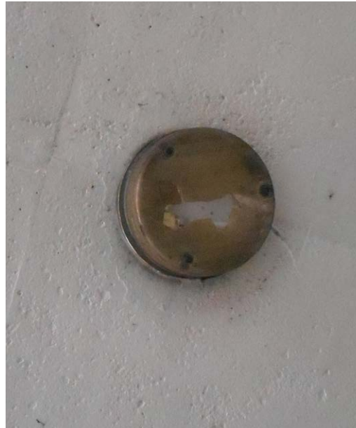
Light in the ceiling- Category 1. (Assumed as the original fitting)
